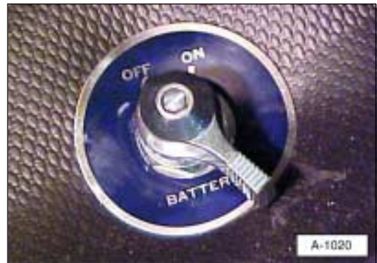
Illustration 10a. Cut-off switch mounted in cab of truck.
