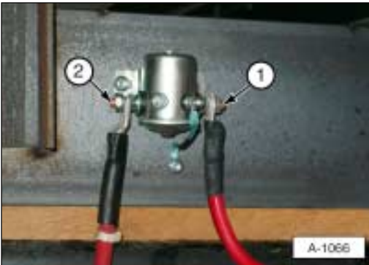
Power cut-off solenoid.
